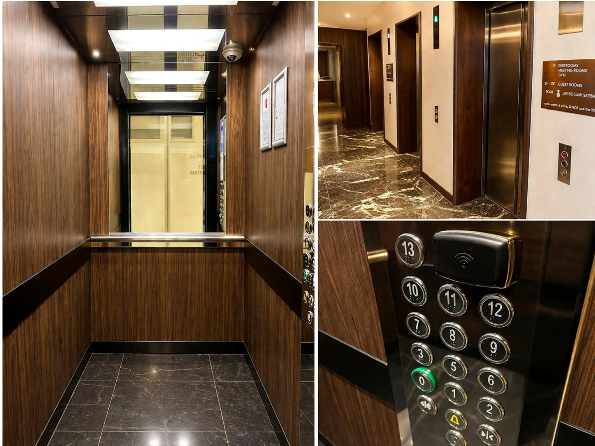
Passenger lifts showing lift interior space, lift lobby access and tactile/Braille control buttons positioned at an accessible height.
